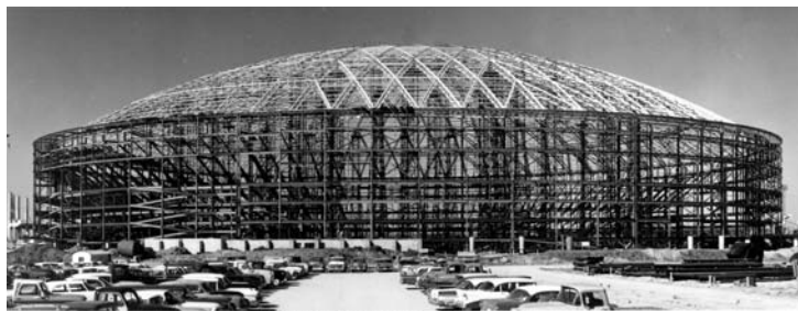
The Astrodome under construction in 1963—Judge Roy Hofheinz, pictured here, was the driving force behind the domed-stadium concept.
